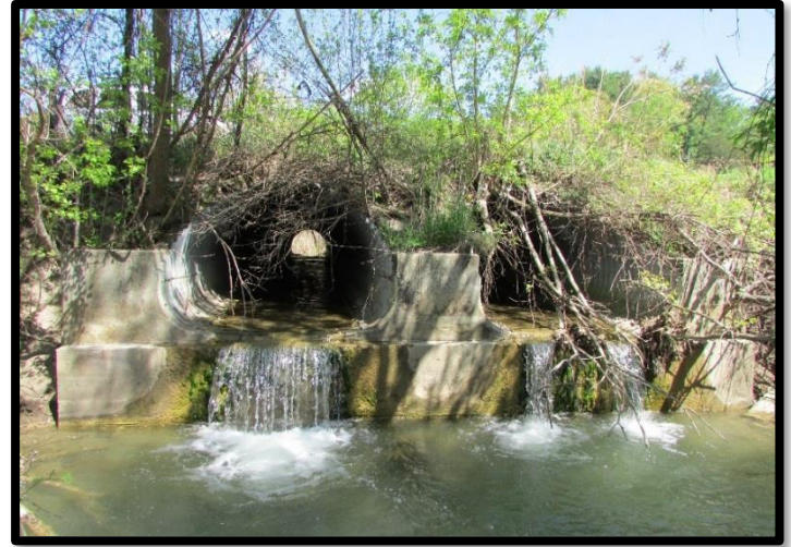
Culverts such as this these can constrict the natural flow of the stream, have a perched outlet that only strong swimmers can jump and contain no natural streambed.
