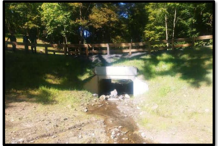
Scenic Hudson Land Trust received a grant to improve the aquatic organism passability and reduce the flooding hazard of this vital piece of infrastructure.
