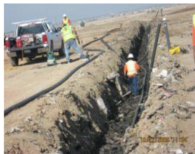
Figure 8: Landfill Application – Gas collection system
