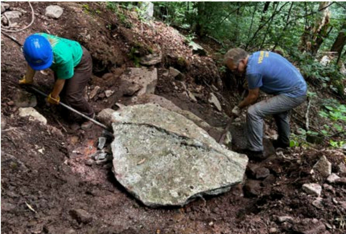
Stewards and Andy Garrison move a large rock on the Phoenicia-East Branch Trail
