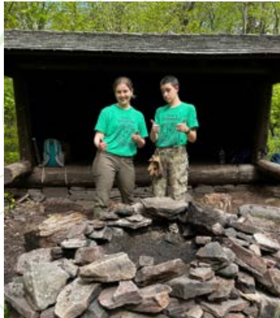
Stewards Tori and Sav show off the newly restored fire ring at the Batavia Kill lean-to
