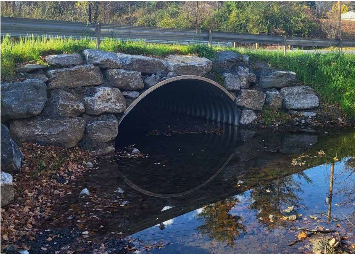
On George Road in the Town of Ghent, a culvert that created a barrier to fish movement was replaced with a bridge on a tributary to Black Creek.
